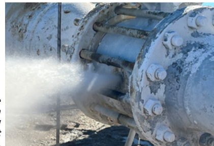
The existing control valve experienced severe erosion and media leaks, requiring frequent replacement and costly downtime.
