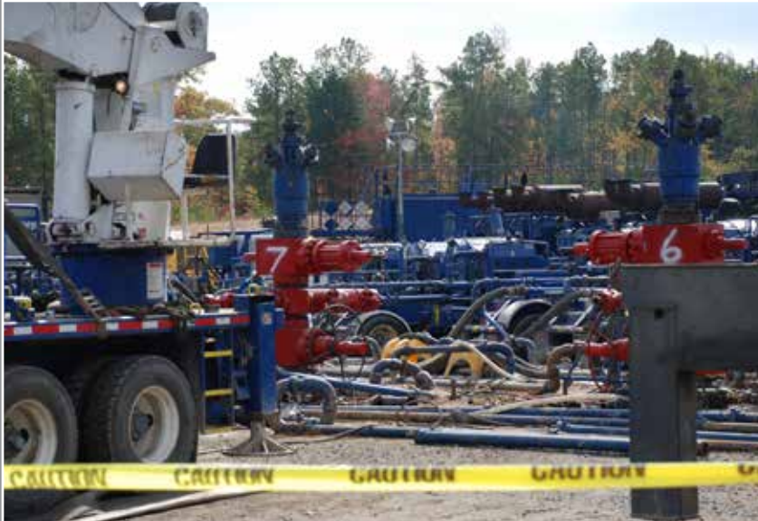
Well heads (numbers 6 and 7) at a drill pad in the Fayetteville Shale gas play of Arkansas.
