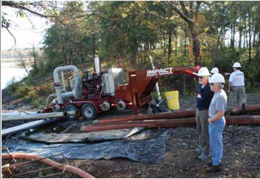
Equipment set up to pump water from a lake to an impoundment for hydraulic fracturing in the Fayetteville Shale of Arkansas.
